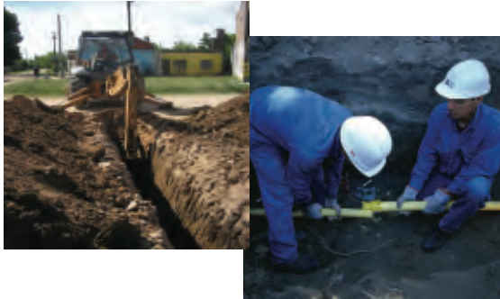
Gas network infrastructure building
